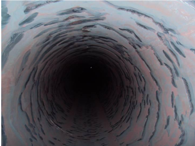
Figures 1: Pipe surface corrosion-erosion
